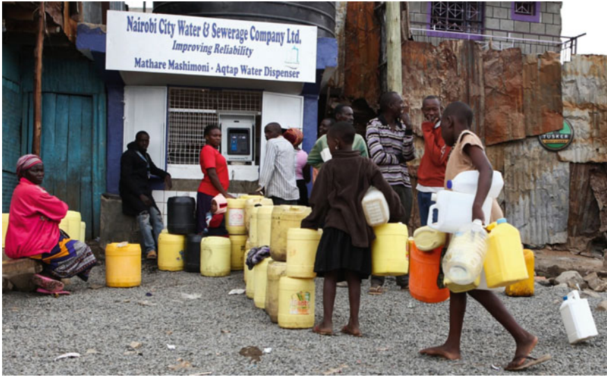
Fig. 24.9 Water dispenser installed in Mathare Slums, Nairobi. Source [37]
