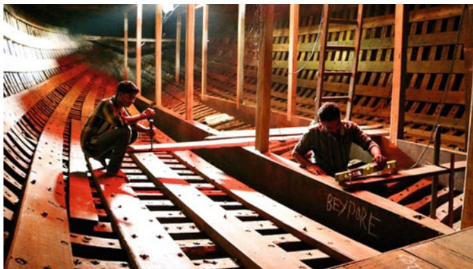
Fig. 17.17 An inside peak into the art of dhow-making. Source Indian Express, published: 19 March 2015, Kerala
